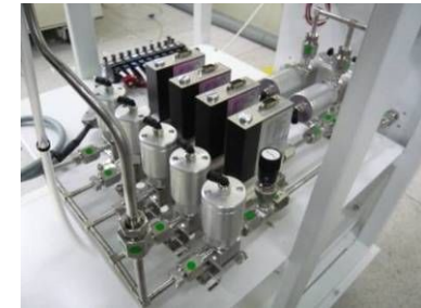
< Gas Delivery module >
