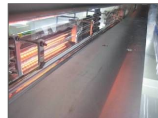
< Heating unit view >
